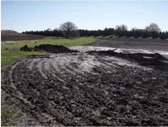
Figure 5. Area of the broken tile. Soil was removed to reach the tile.
