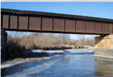
Ice melt in Straight River from straight pipe outlet.
